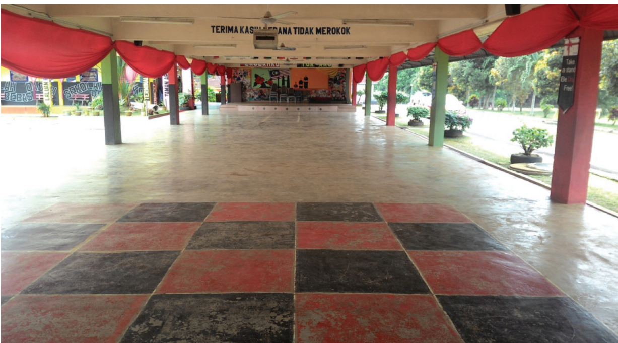
Figure 3: Dust deposited on floor of the school
