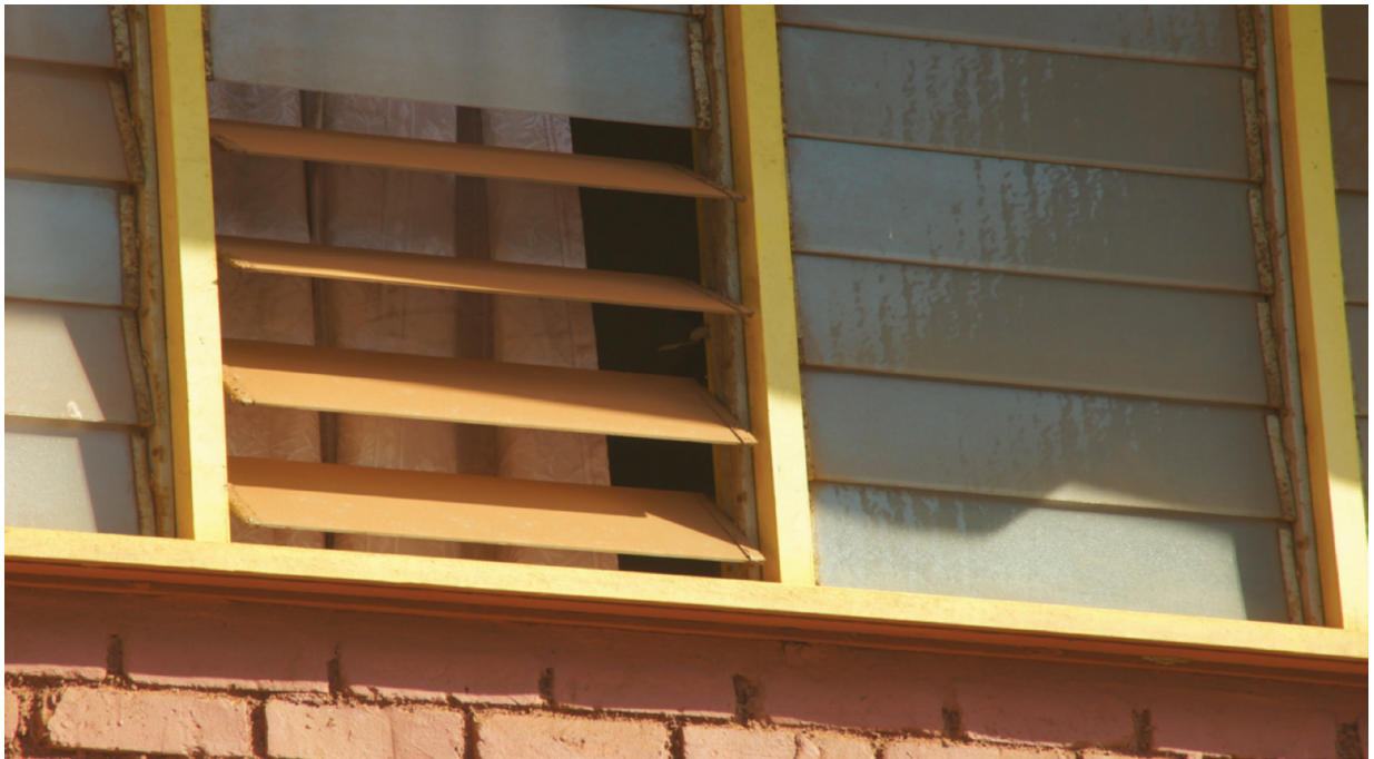
Figure 4: Red dust deposited on window of quarter next to Kuantan Port
