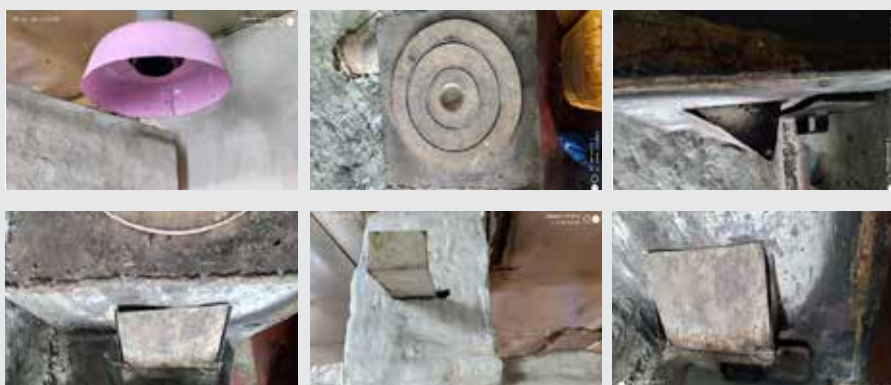
Picture 2. The stove and chimney condition of case two household
