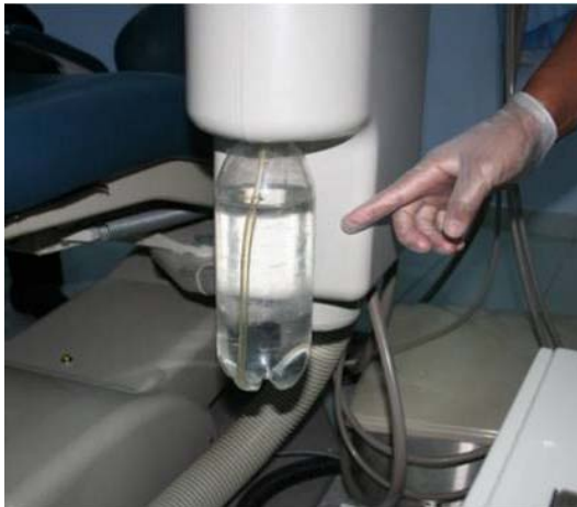
Fig. 1 The source of water in DUWLs from the independent water reservoir (bottle).
