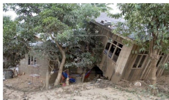
Figure 7: Property damaged: House on a house.
