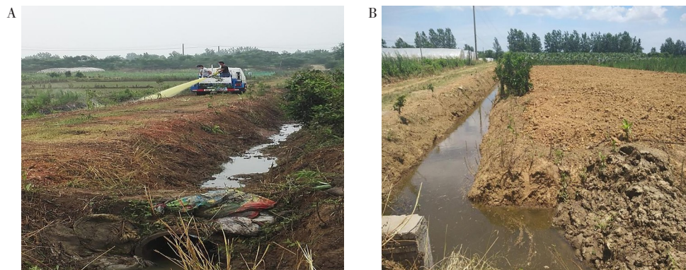
A. 灭螺前;B. 灭螺后。A. Before engineering snail control; B. After engineering snail control.
