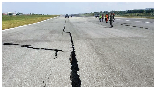
Figure 1. Mutiara airport runway cracked, and only small propeller aircraft and military airplanes could land.
