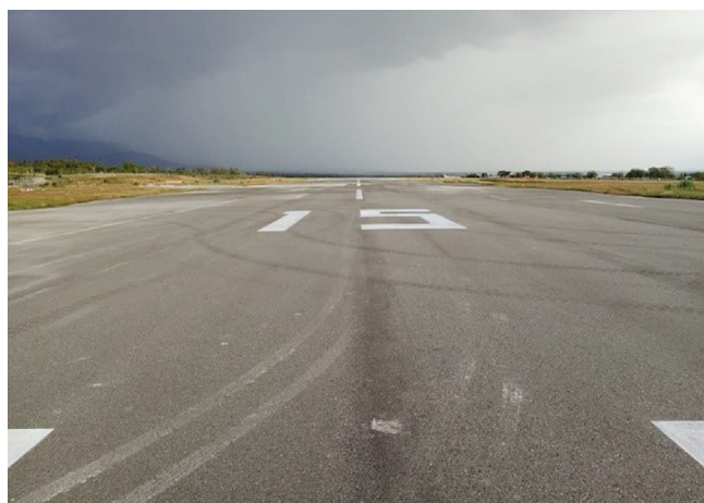
Figure 3. Section of runway 15 repaired over two weeks, allowing Airbus and Boeing narrow-body aircraft to resume operations.
