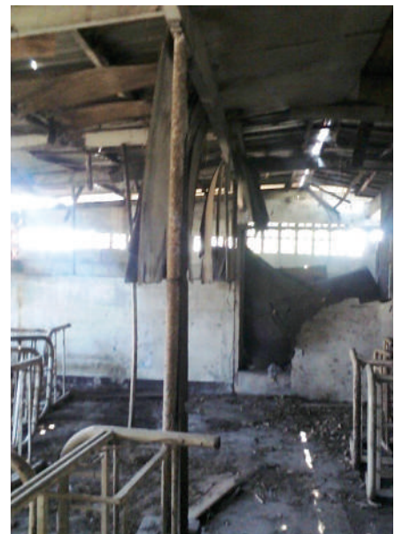
Figure 8. Former mercury storage area with leaking roof and adequate ventilation.
